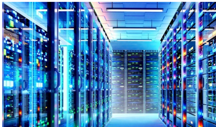
Data centres are already consuming vast amounts of electricity and the prediction is that this will grow enormously.
